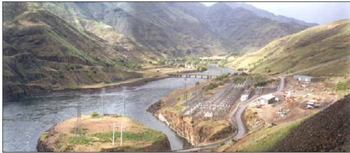
Fig. 11. Substation facilities at Brownlee Dam.
