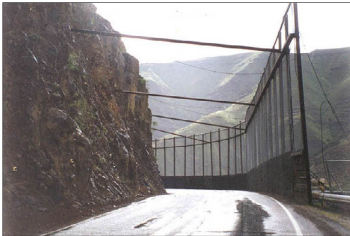
Fig. 13. The Brownlee Cage protects Project facilities on the approach to Brownlee Dam.
