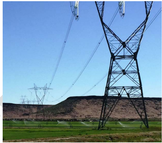
500-kilovolt (kV) transmission line near Melba, Idaho.
