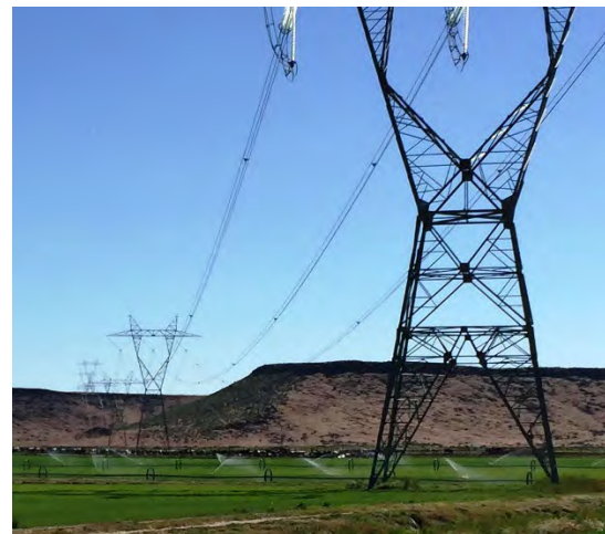
500-kilovolt (kV) transmission line near Melba, Idaho
