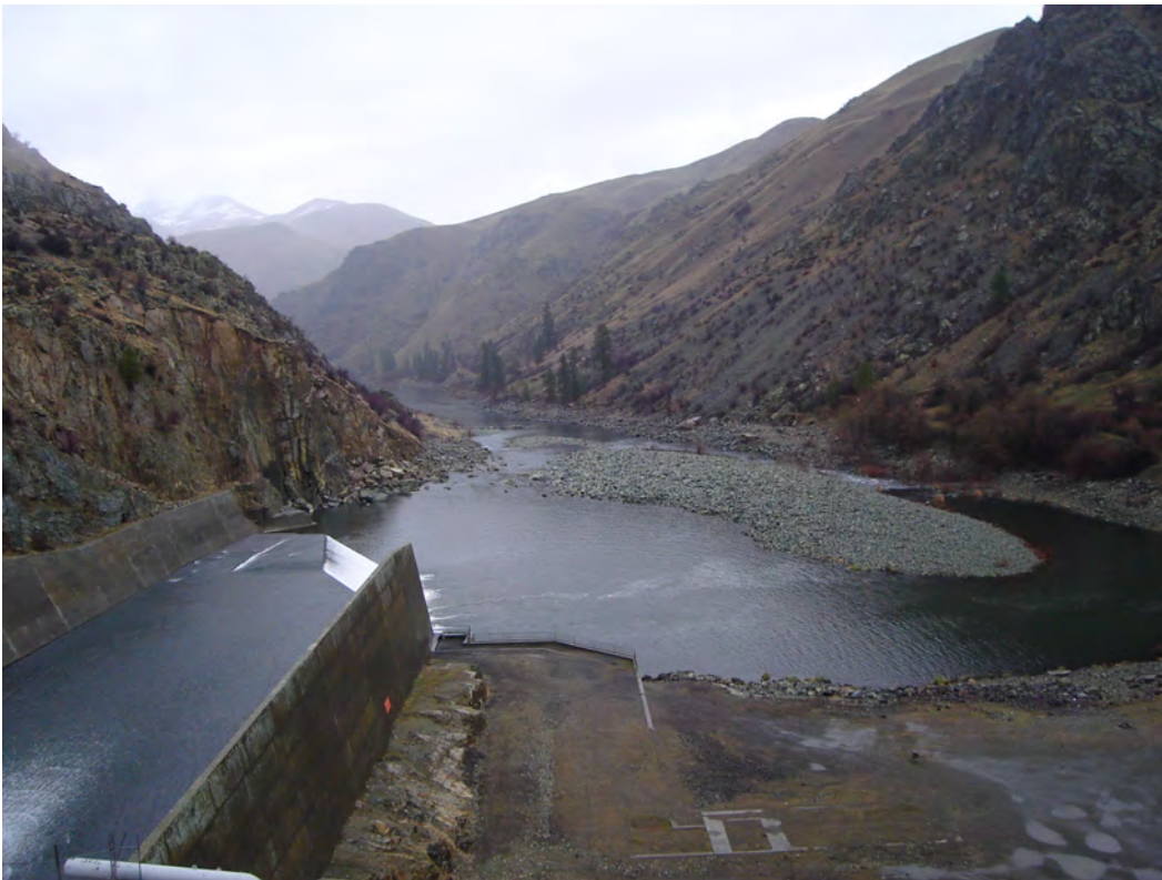
Photo 1.3 Material deposition downstream of spillway.
