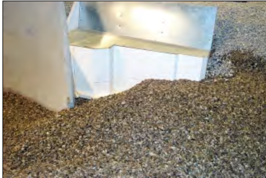
Figure 4.14. Fish ladder entrance erosion after 20 kcfs per sluiceway bay
