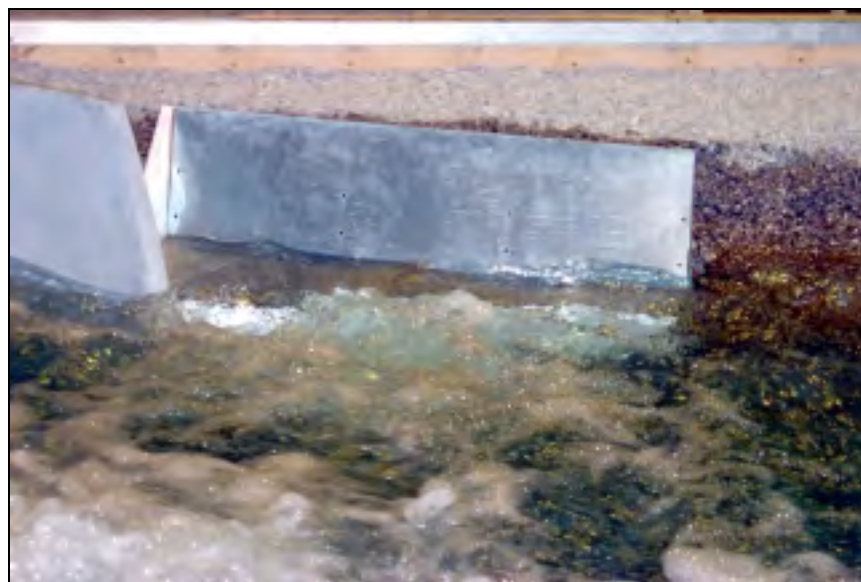
Figure 4.40. Waves breaking on fish ladder entrance during 50 kcfs per crest gate
