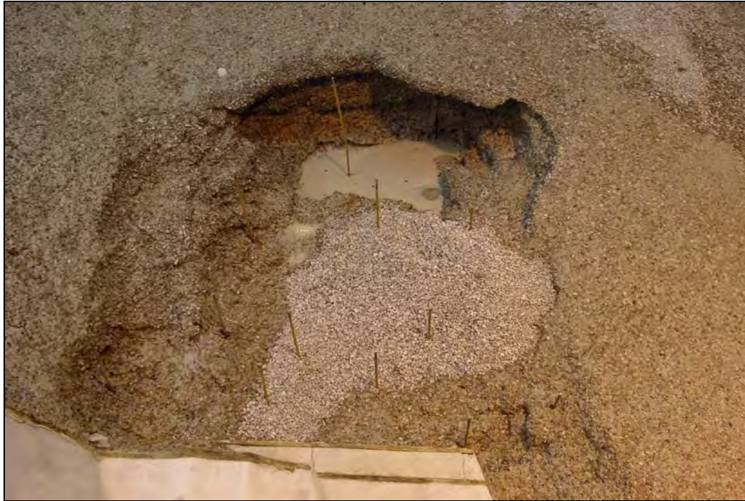
Figure 4-9. Primary scour hole looking downstream from apron after the scour test with deflector (IP-3D-14)
