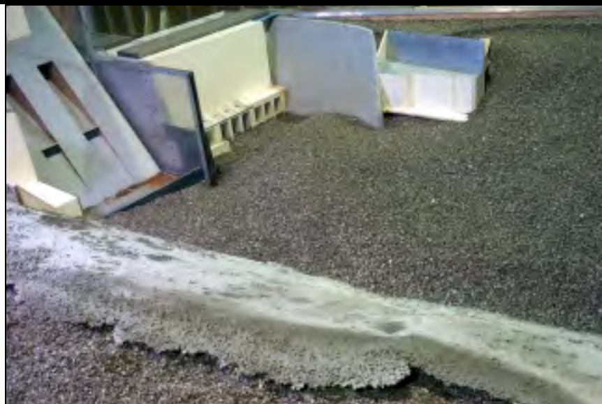
Figure 4.68. Erosion patterns near powerhouse and fish ladder entrance
