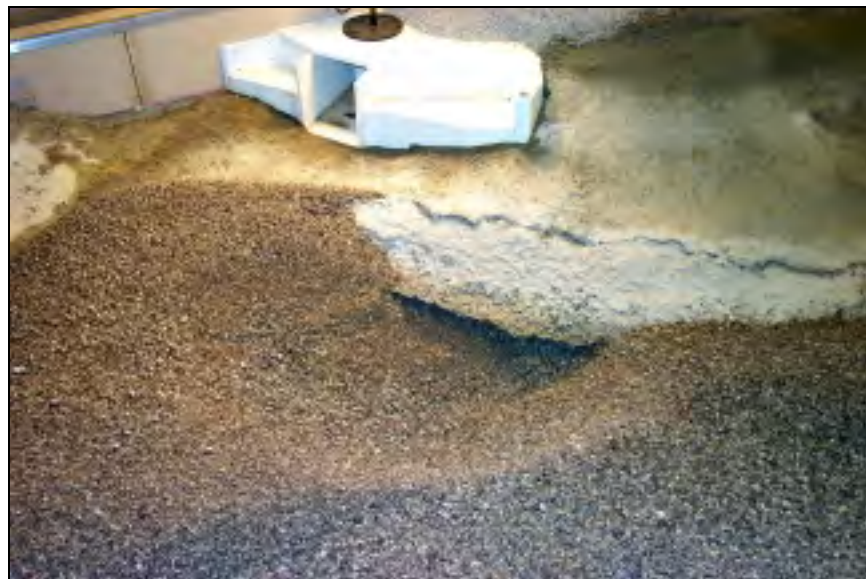
Figure 4.32. Tailrace scour after 30 kcfs per crest gate
