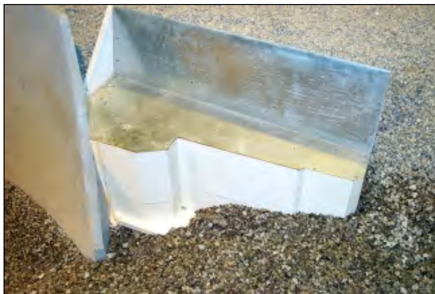
Figure 4.10. Fish ladder entrance erosion after 15 kcfs per sluiceway bay
