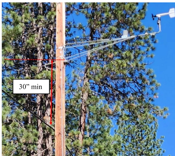
Weather Station with Communications
