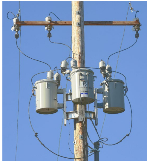
Figure 5 Three-phase Overhead Transformers
