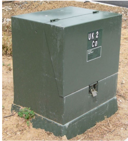
Figure 7 Other Padmounted Equipment -Not a transformer
